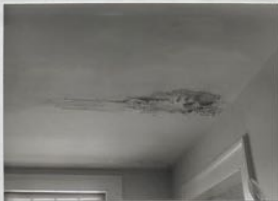
Photograph 70 Ceiling of upstairs hallway of Chaise House. Severe damage is being caused by leakage down from the attic, probably due to failure in the roofing.
