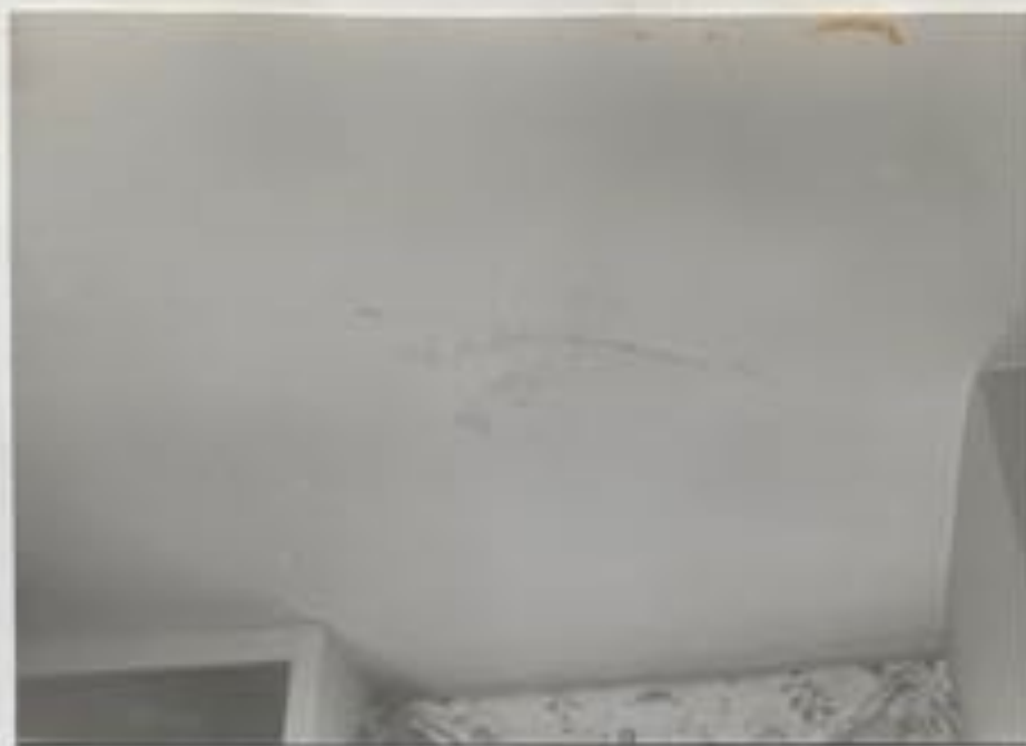
Photograph 69 Ceiling of south west chamber, south of the chimney, showing stains and crack from leakage around chimney.
