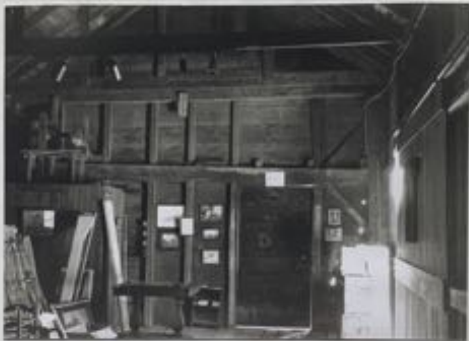
Photograph 19 North wall of the Corn Barn. This was left intact when the structure to the south was rebuilt in 1928.
