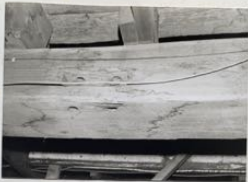
Photograph 60 Close up of circular sawn beam, reused as a girt under the reconstructed sheds of 1928. Also shows old mortise and peg holes.
