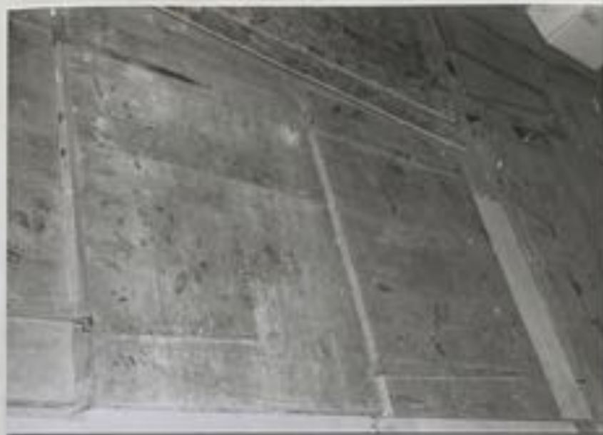
Photograph 18 Possible stall doors, found in the attic of the Porter-Phelps-Huntington House wood shed.
