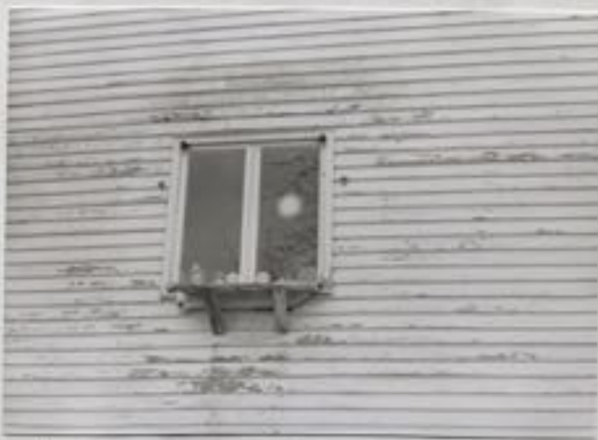
Photograph 66 Close up of rear (west) wall of Chaise House, around kitchen window, showing severe paint deterioration and damage to bare clapboards underneath.
