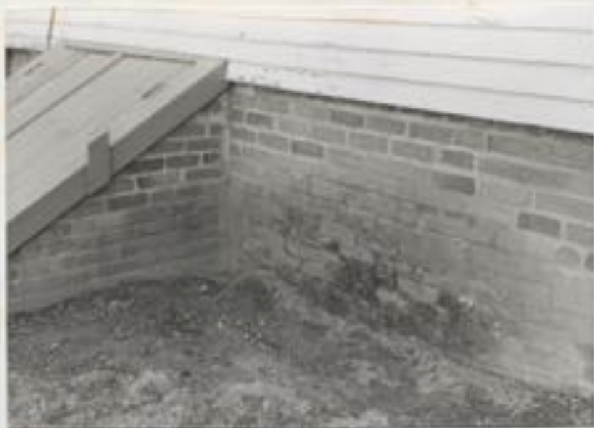
Photograph 67 Rear foundation near Chaise House bulkhead, showing moss growing on the brick.
