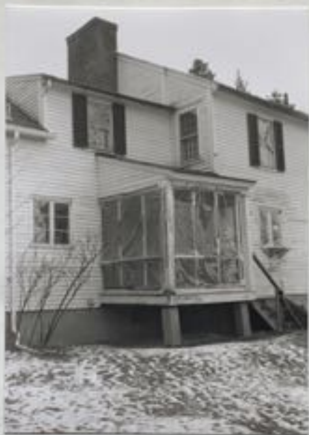
Photograph 41 Close up view of porch at north west corner of Chaise House, 1989.
