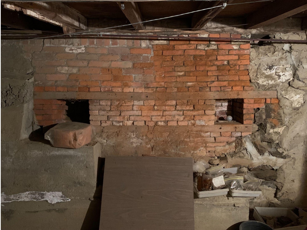
Figure 22: West face of 1771 Ell chimney (below the Keeping Room, see figure 3.1) in cellar of Forty Acres Main House (HAD.319) showing brick shelving units, camera facing east.
